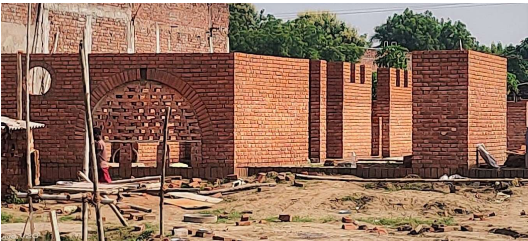
The arch and a circular window are in place. The west interior wall vents are in progress.
